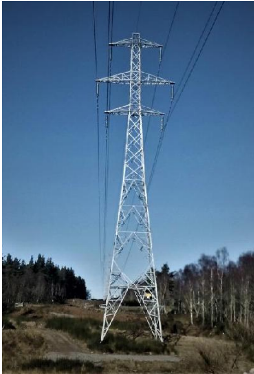
Plate 2.2: Example Steel Lattice Tower OHL Structure
