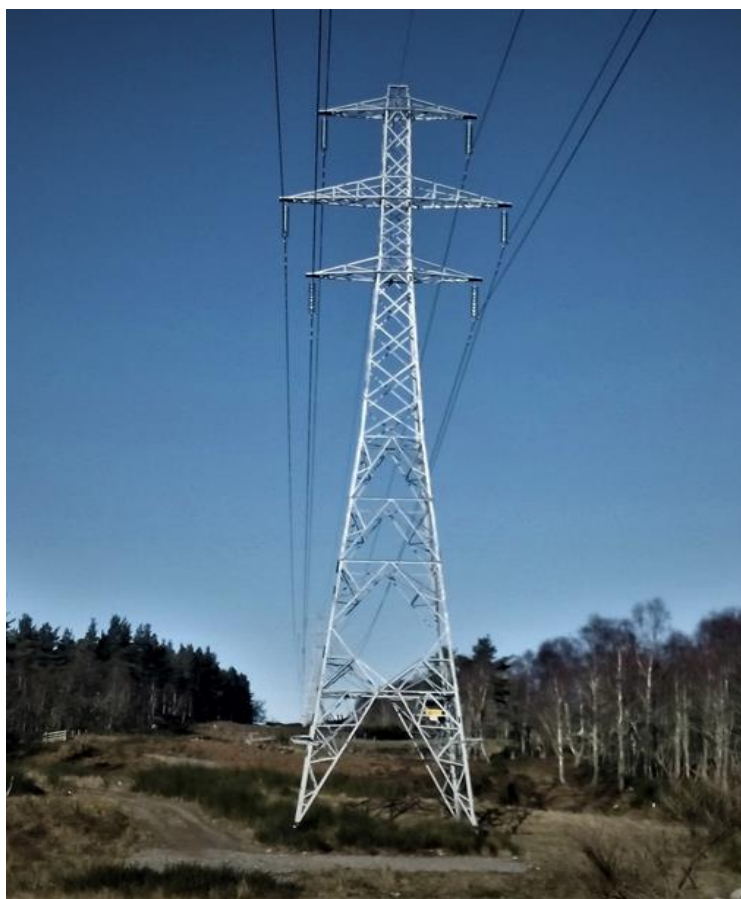
Plate 2.1: Example Steel Lattice Tower OHL Structure
