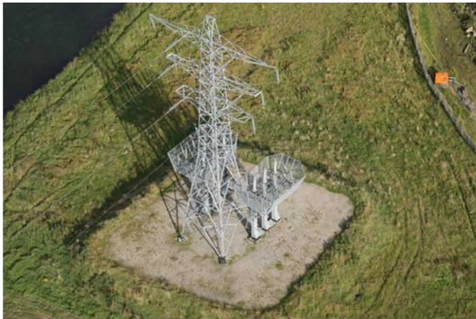
Plate 2.3: Typical Cable Sealing End Tower
