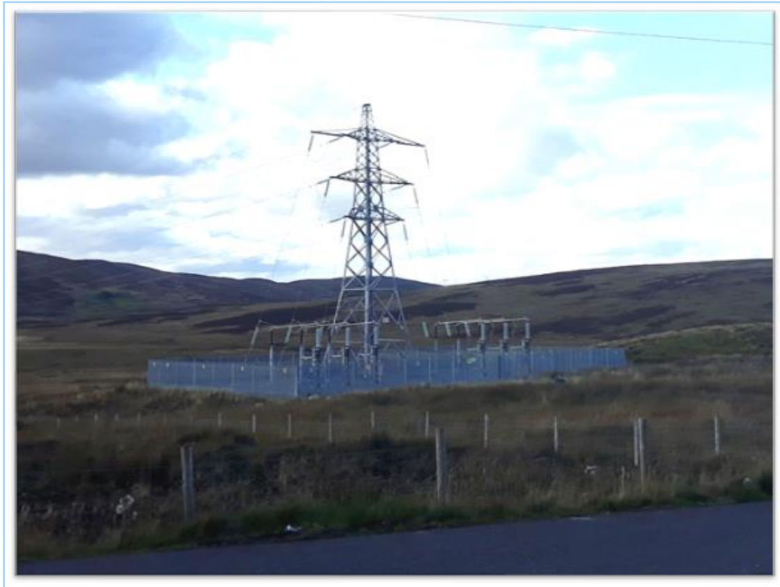
Plate 3.5: Example of a Cable Sealing End Compound
