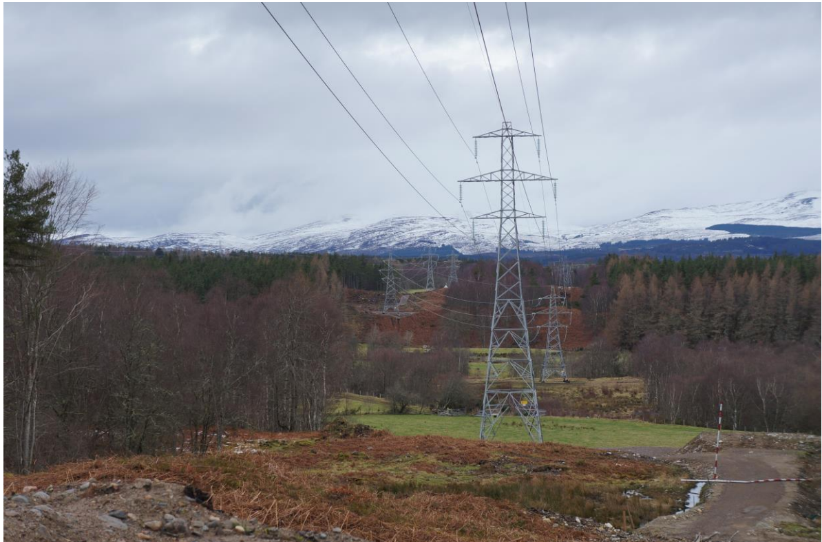
Plate 3.1: Photograph of Steel Lattice Tower Double Circuit (L7 series)
