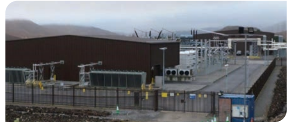
Existing Melgarve Substation
