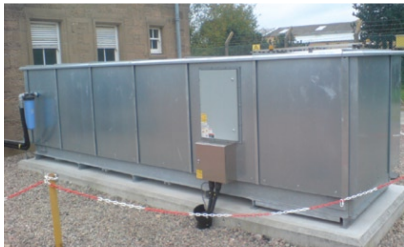
Figure A5.1 – Flow Battery Trial, Nairn substation
