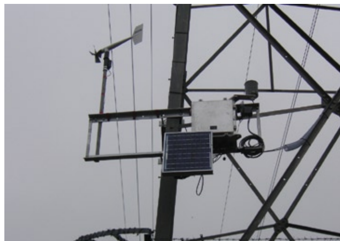
Figure A5.2 – Dynamic Line Rating technology
