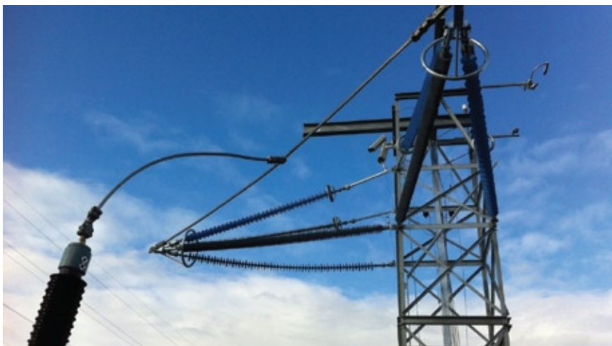
Figure A5.5 Installation at St Fergus Switching Station
