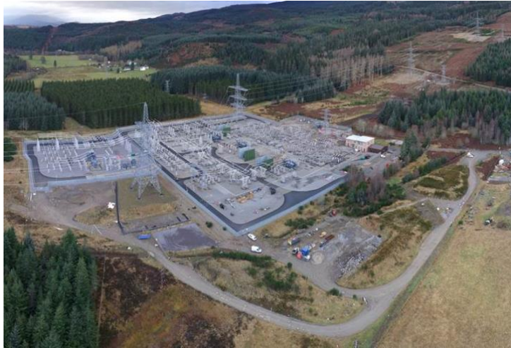
Figure 5 Fort Augustus Substation
