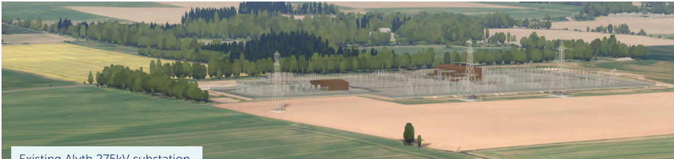
Existing Alyth 275kV substation
