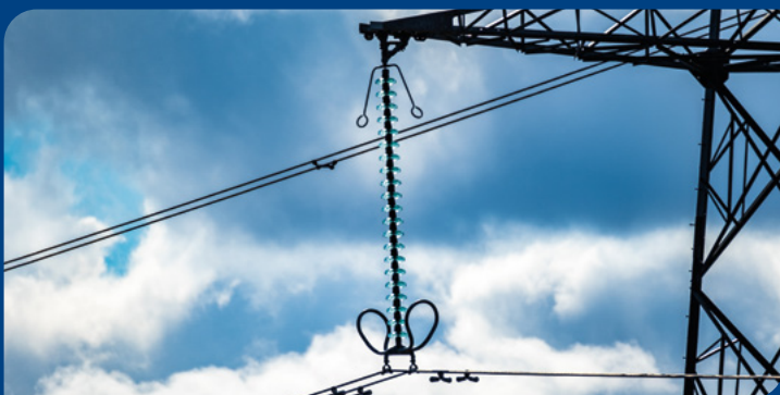
Both circuits of the existing Beauly – Denny overhead line now need to operate at 400kV capacity
