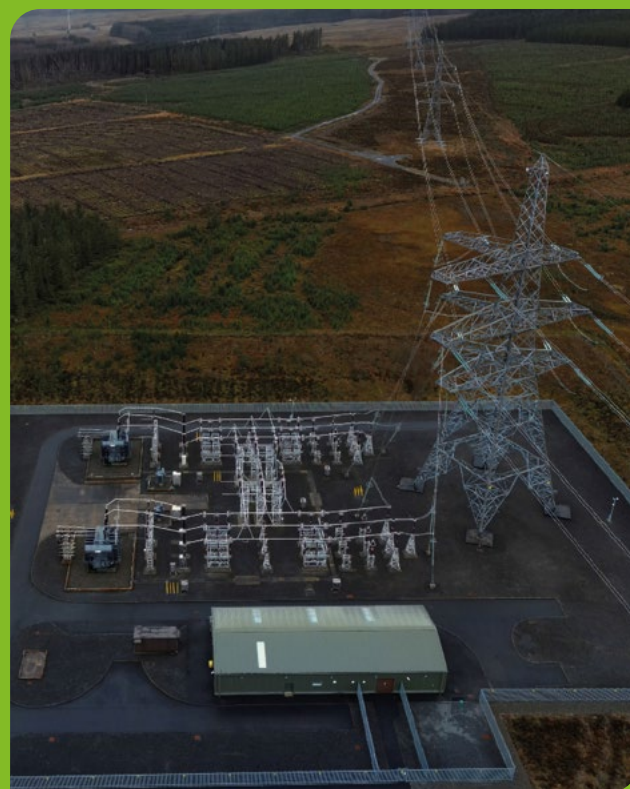
Existing Braco West 275kV Substation
