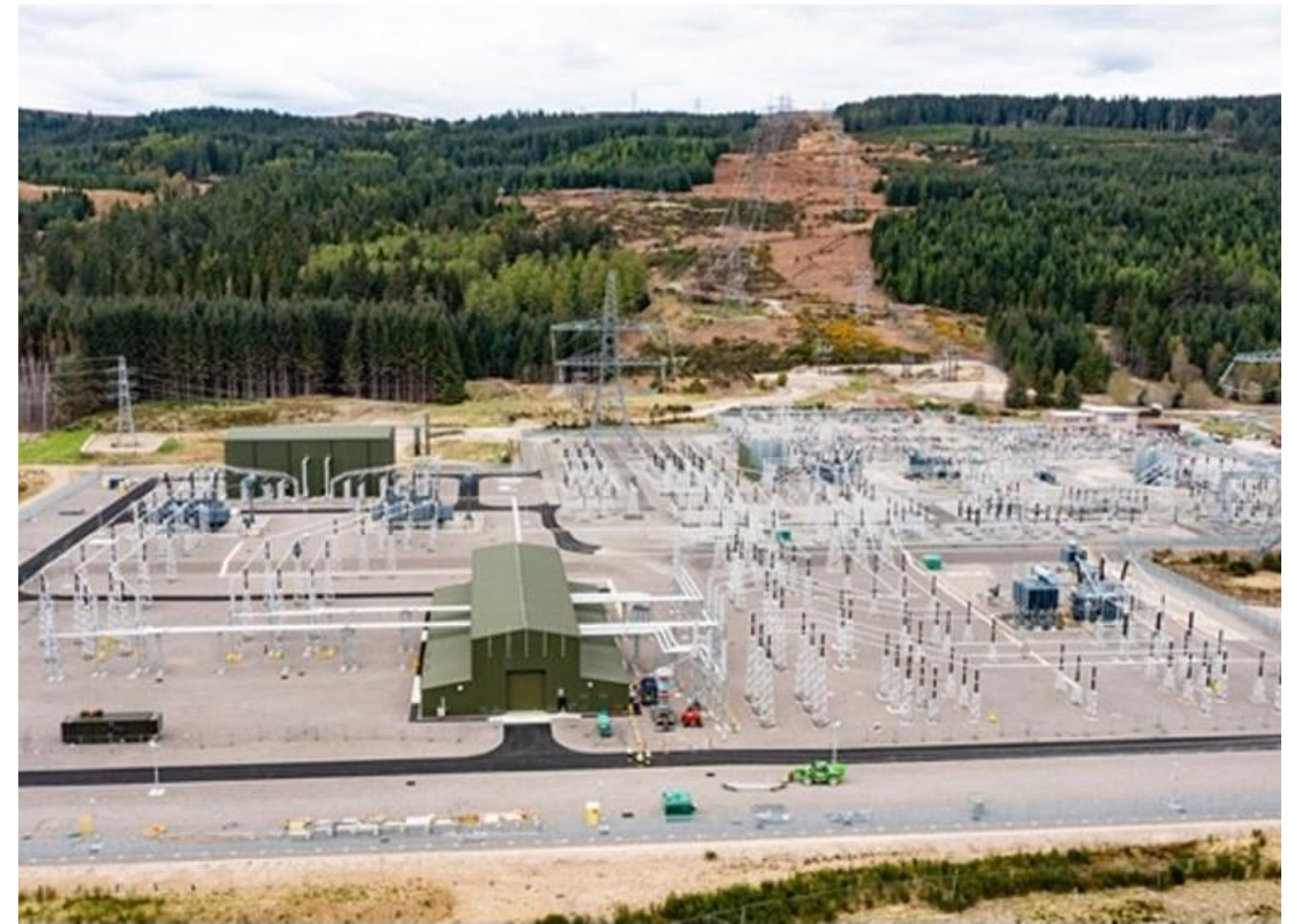
400/132kV substation at Fort Augustus which has a mixture of AIS and GIS technologies
