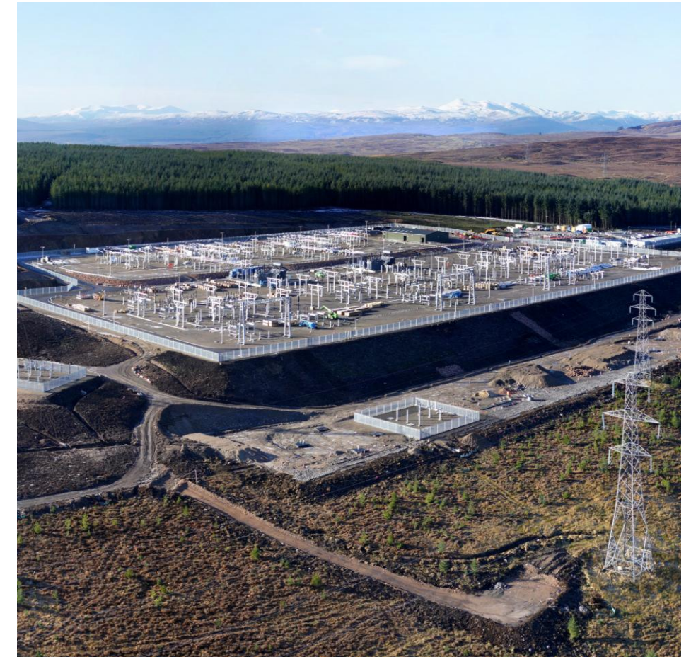
275kV AIS substation at Loch Buidhe
