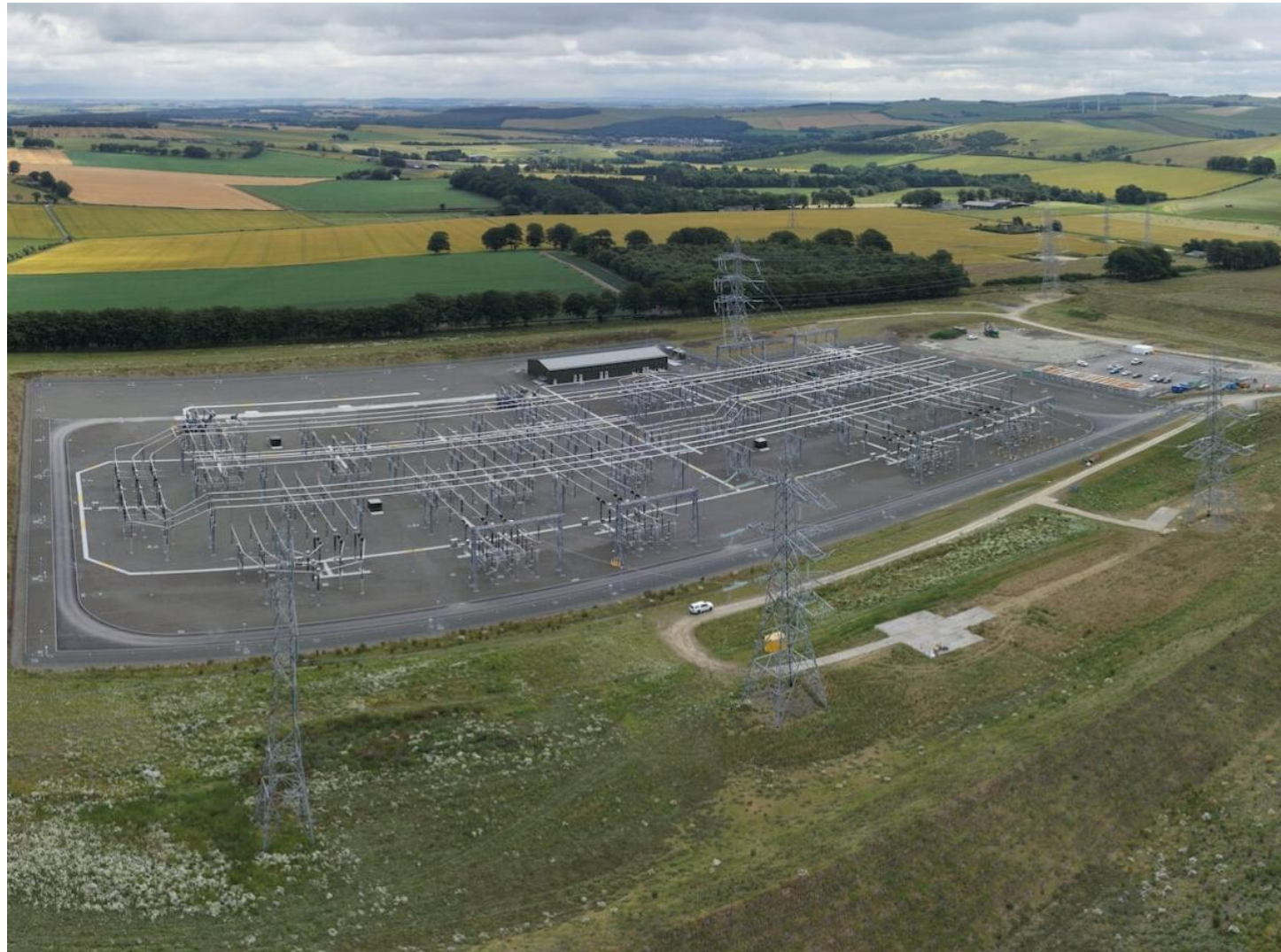
400kV AIS substation at Rothienorman
