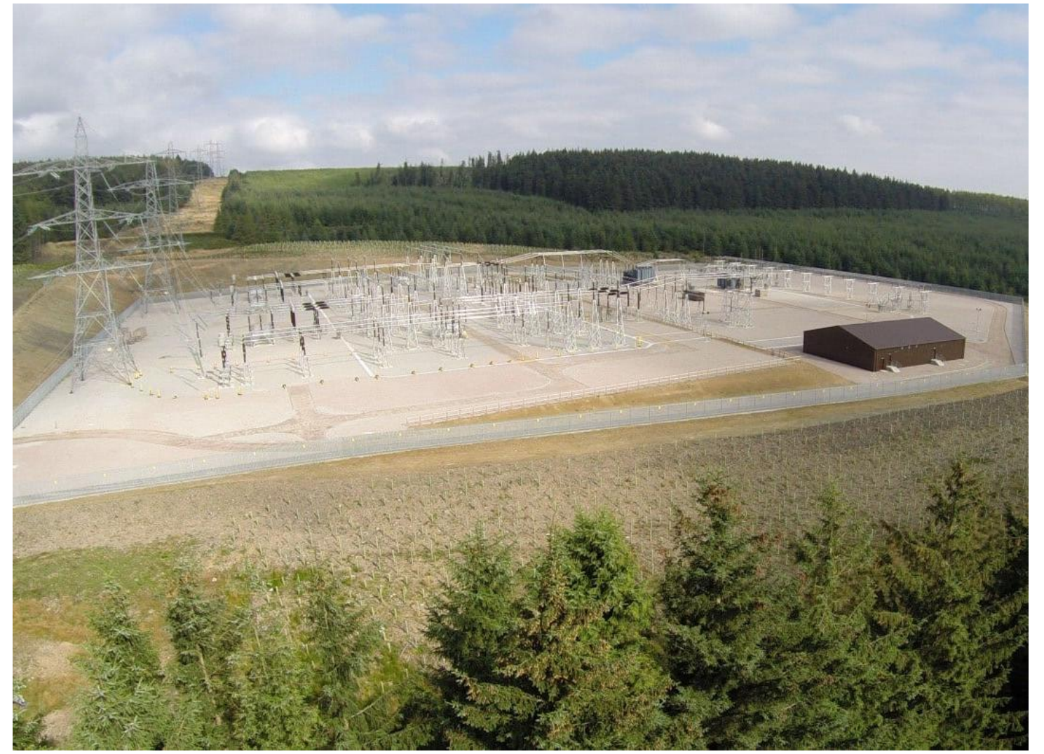
275kV AIS substation at Fetteresso (currently being upgraded to 400kV)
