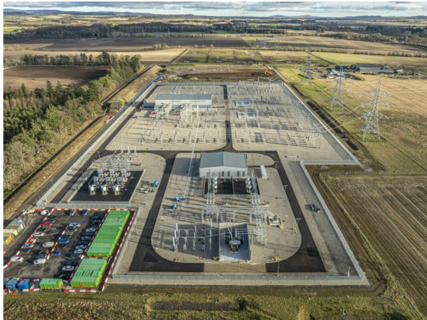
275kV GIS substation at Alyth (currently being upgraded to 400kV)
