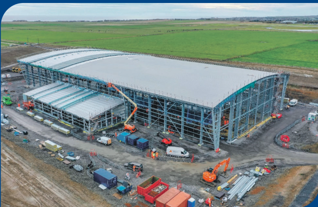
October 2021 roof lining sheets installed with the insulation and top sheet commencing thereafter.
