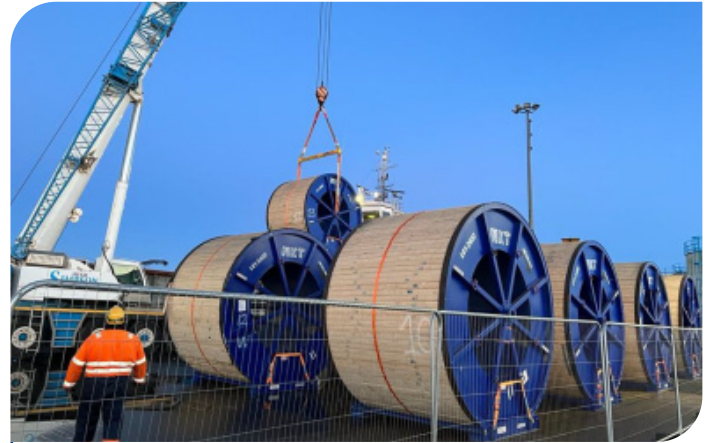
Cable Drums, Wick
