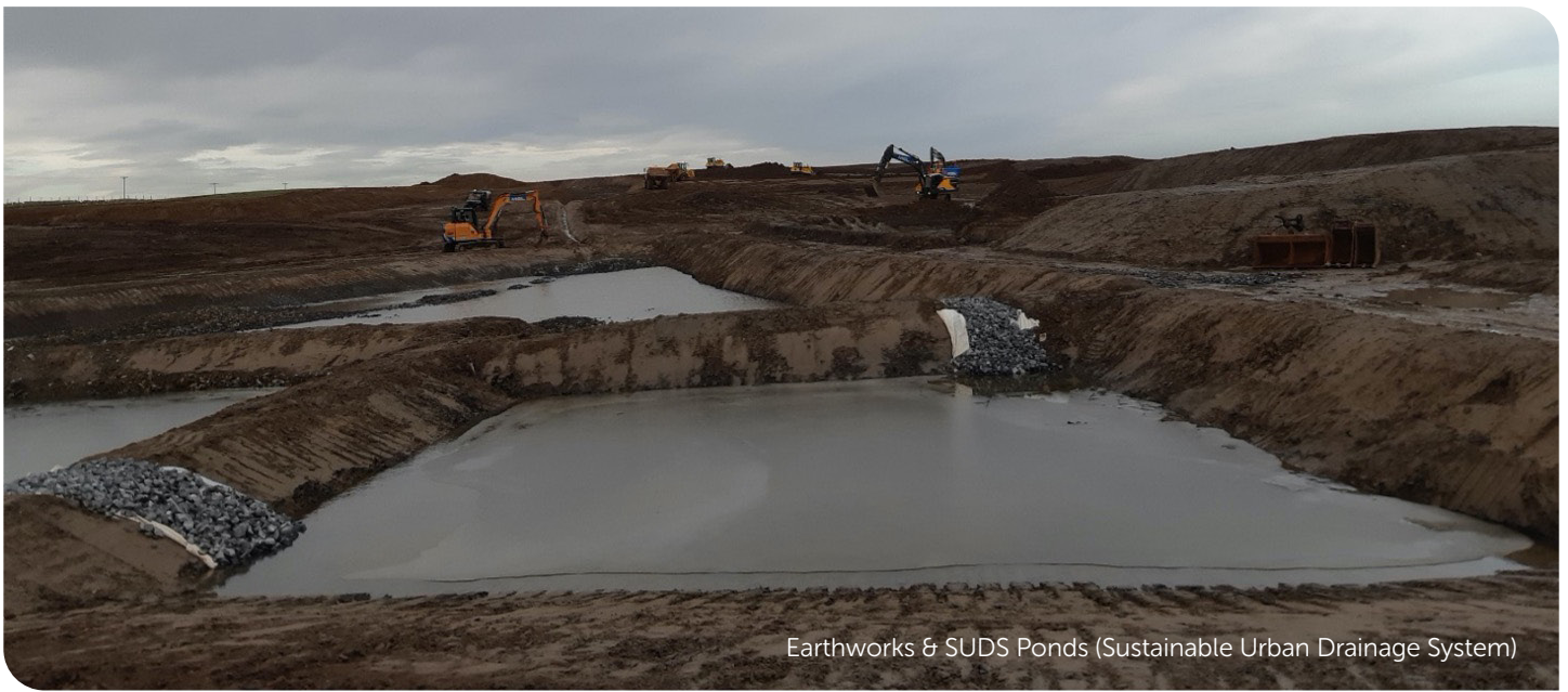
SUDS Ponds (Sustainable Urban Drainage System)
