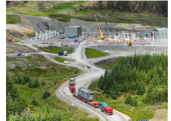
Hauliers approaching the Creag Dhubh substation with an SGT
