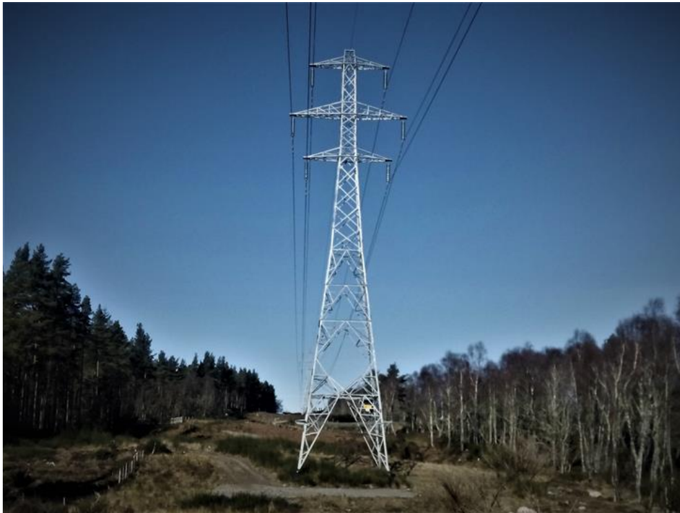
Plate 2.2: Typical Steel Lattice Tower (L7c)
