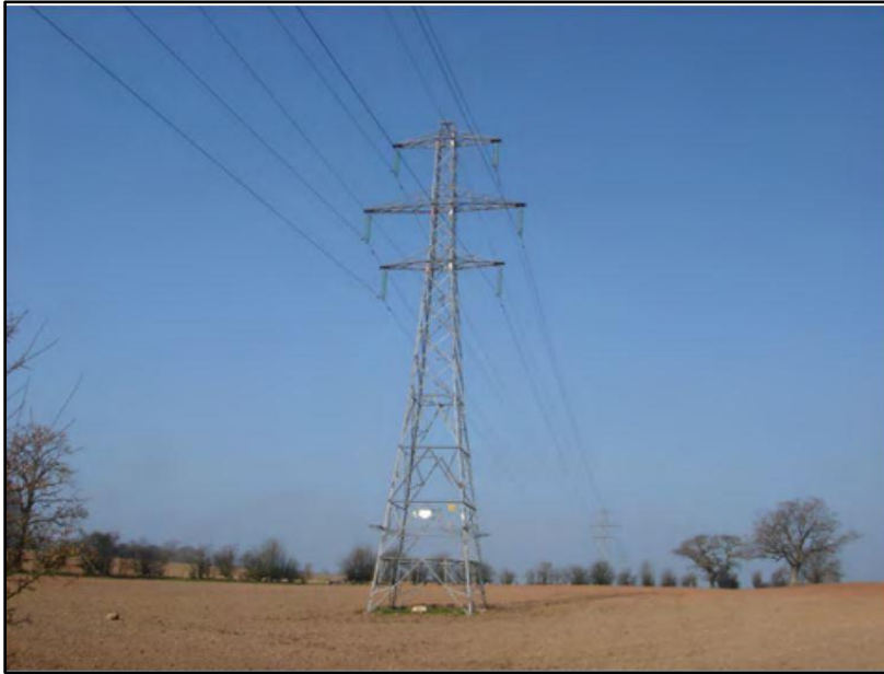
Plate 2.2: Typical Steel Lattice Tower (L7c)
