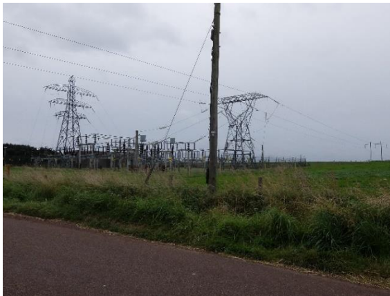
Photo 1: Brechin substation from public road
