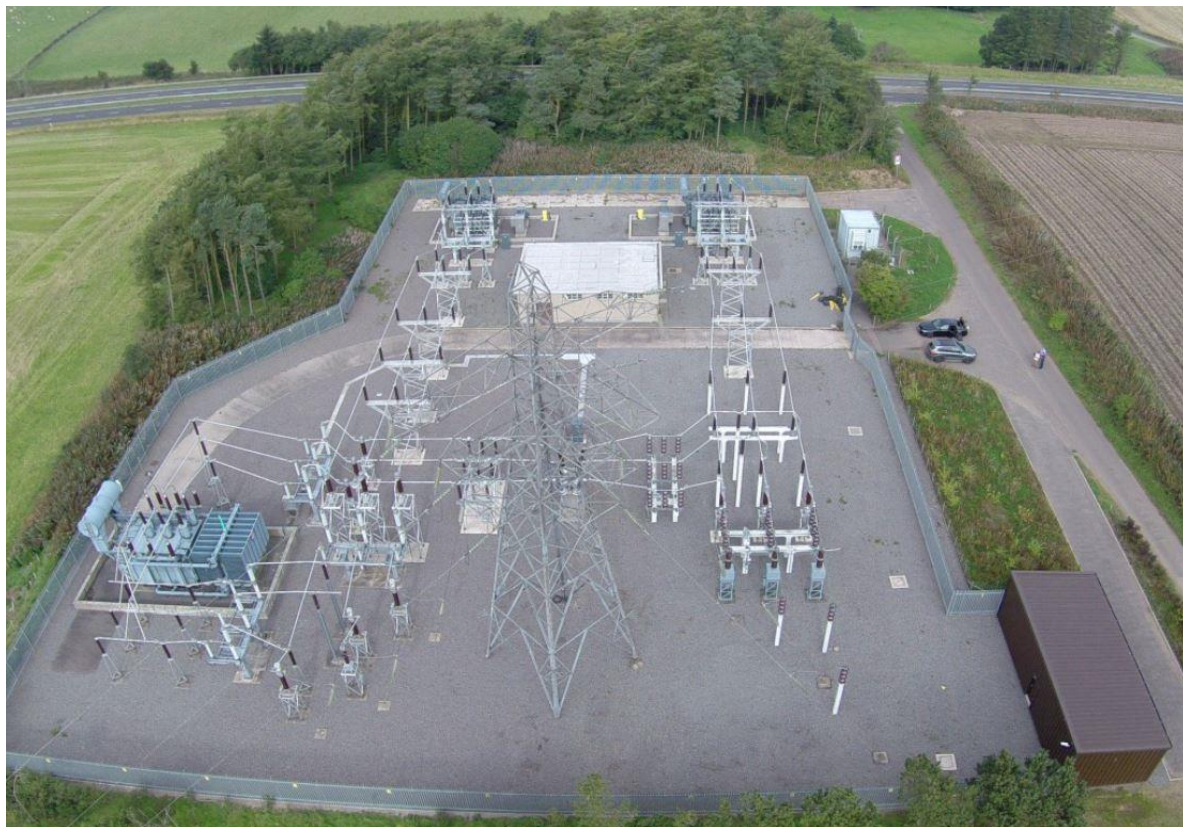
Plate 2.1 - Aerial Photograph of the Existing Fiddes Substation
