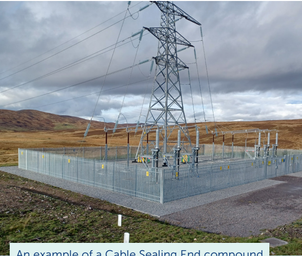
An example of a Cable Sealing End compound
