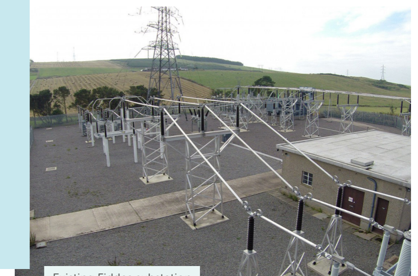
Existing Fiddes substation
