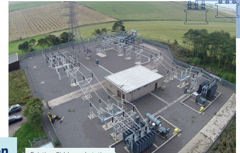
Existing Fiddes substation
