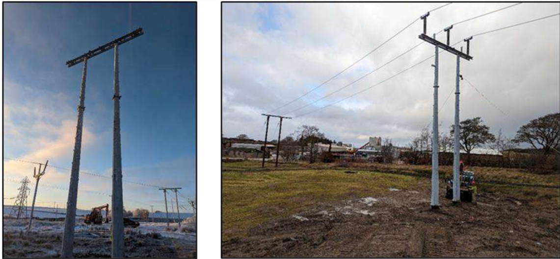
Plate 3.1: Example Steel Trident H Poles
