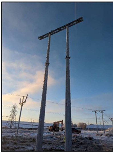
Plate 2.1: Example Steel Trident H Poles
