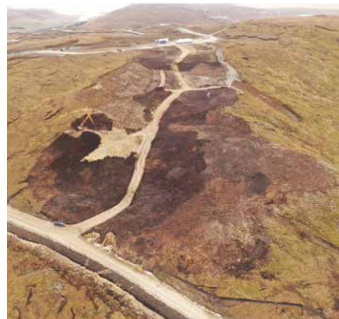
Borrow pit KBP02, West of Kergord. Layers of peat are being applied to exposed rock seams, ahead of final reinstatement.
