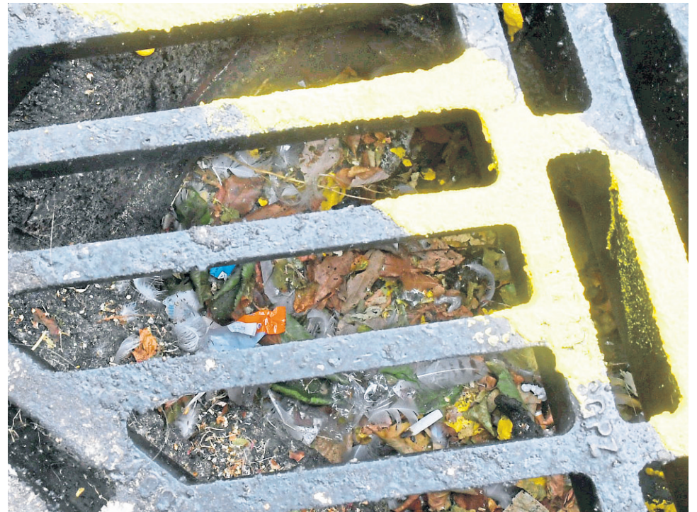
BLOCKED: Fife Council aims to keep gullies clear to reduce the risks of flood damage.
