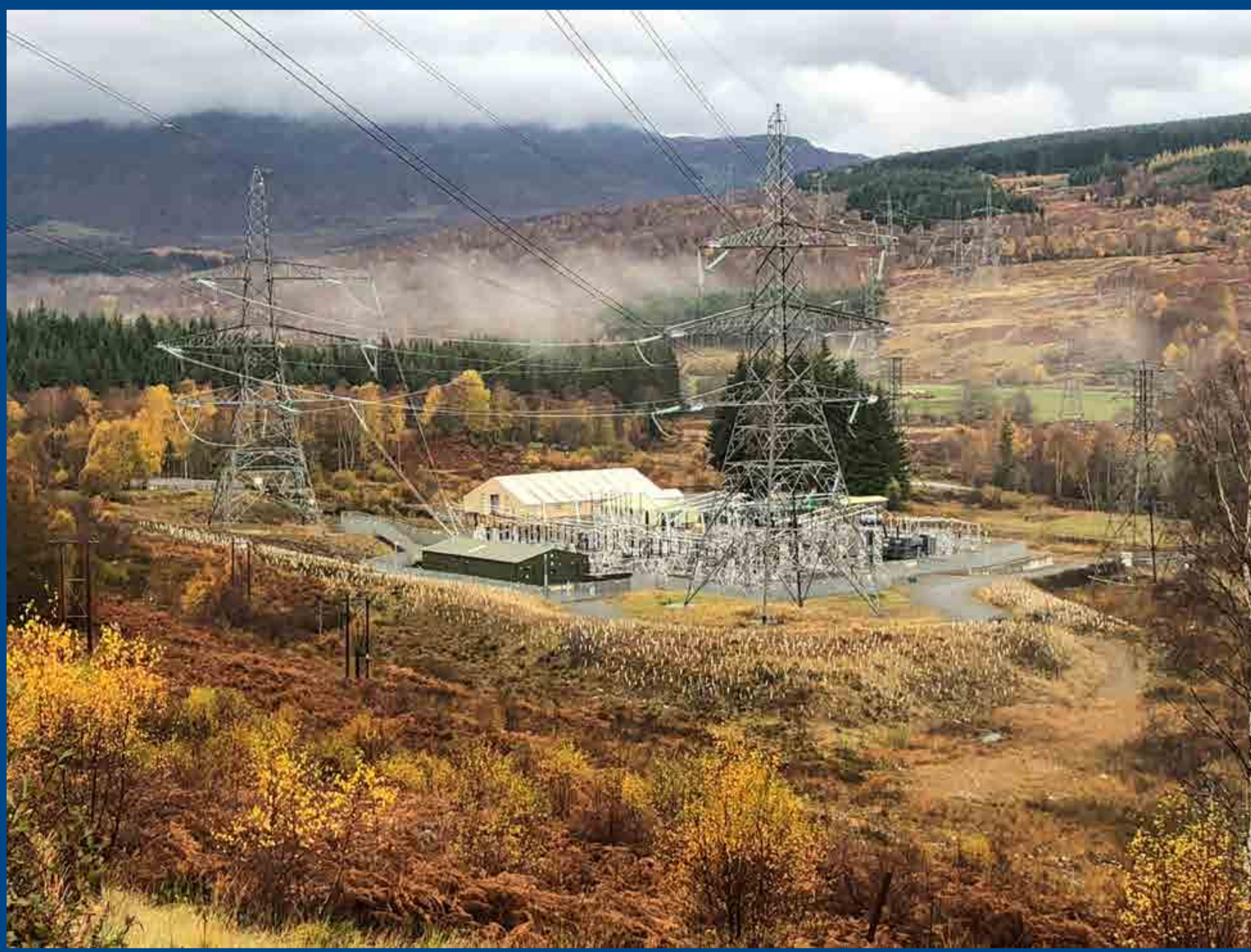
Minor internal alterations to protection and control systems will also be required at the existing 275kV substation.
