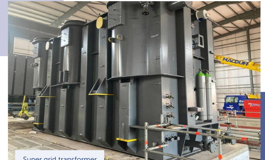
Super grid transformer
