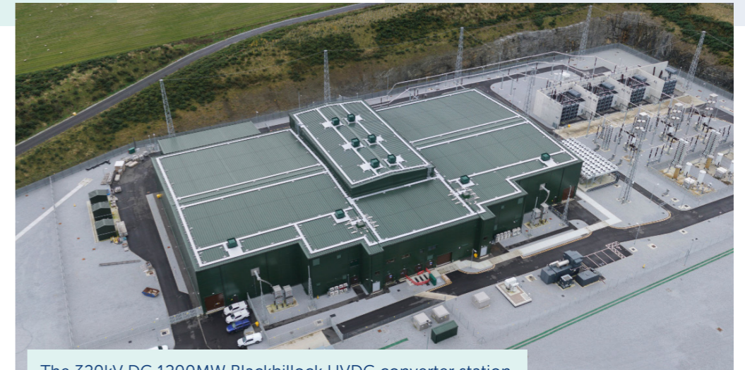
The 320kV DC 1200MW Blackhillock HVDC converter station
