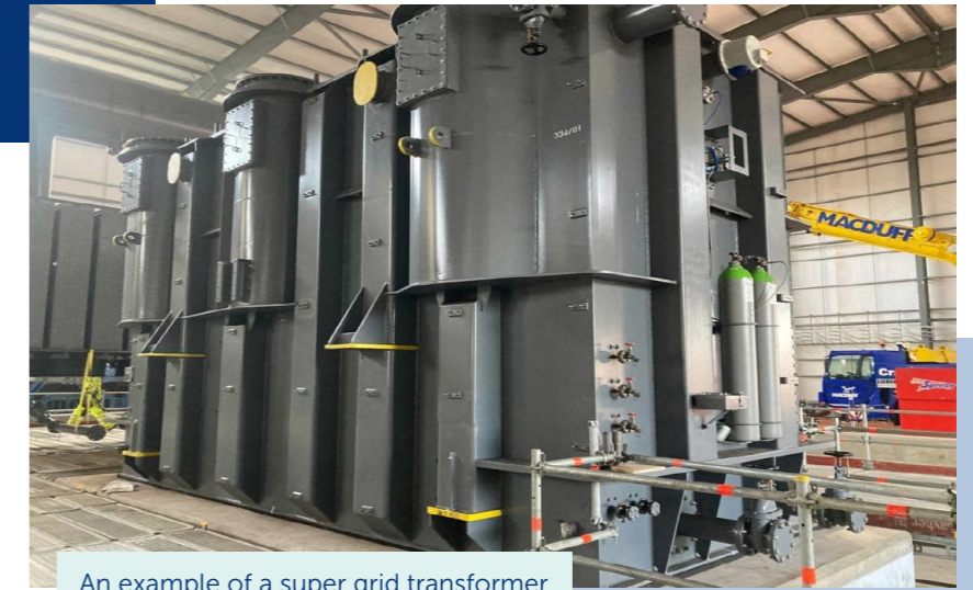
An example of a super grid transformer
