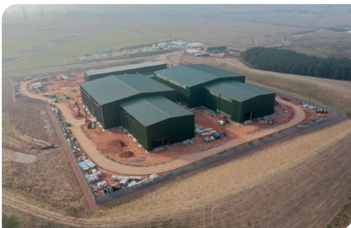
400kV substation at Peterhead
