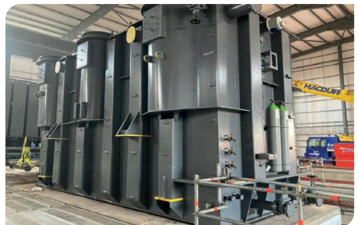
Super grid transformer
