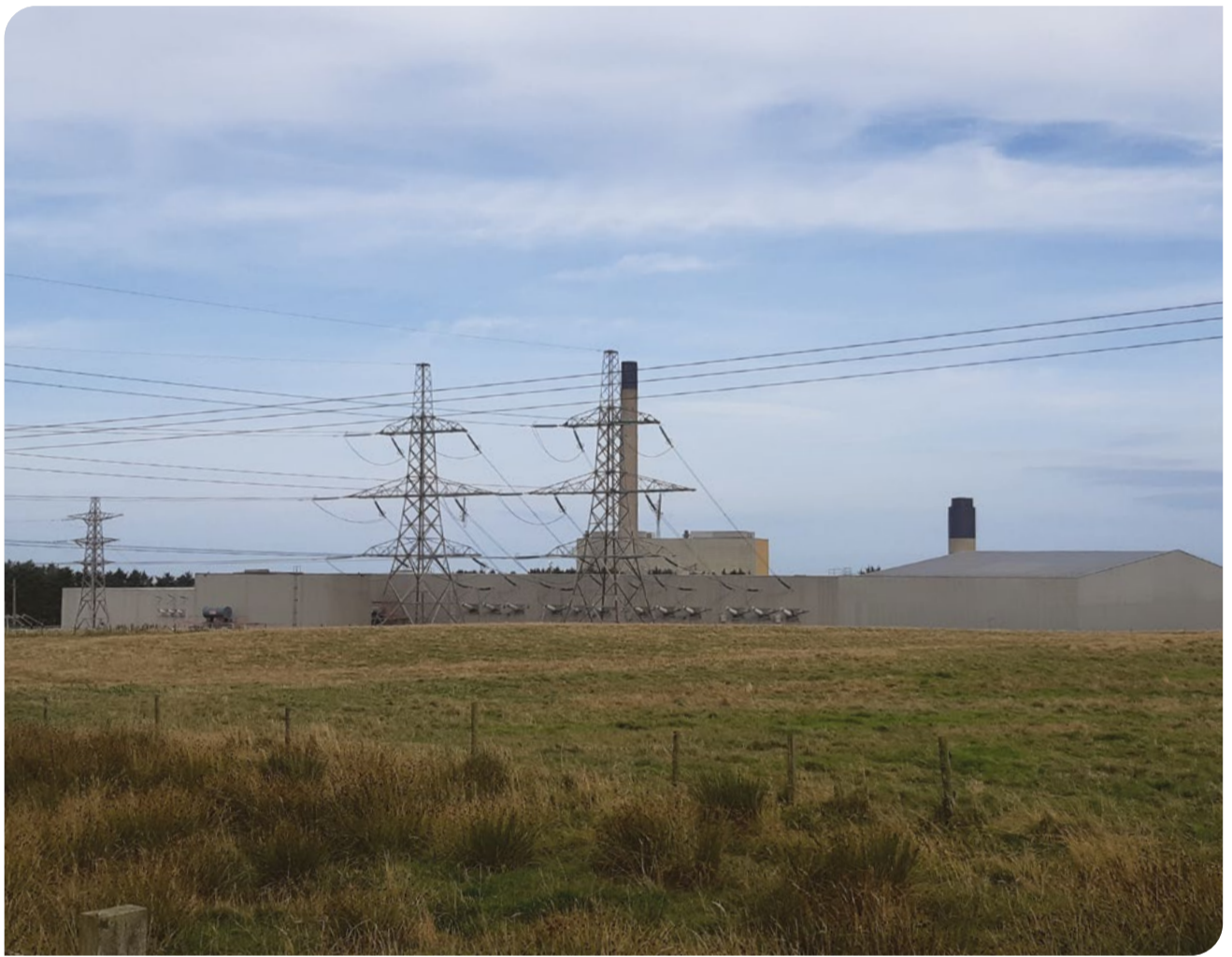
A view of the existing Peterhead 275/132kV substation.
