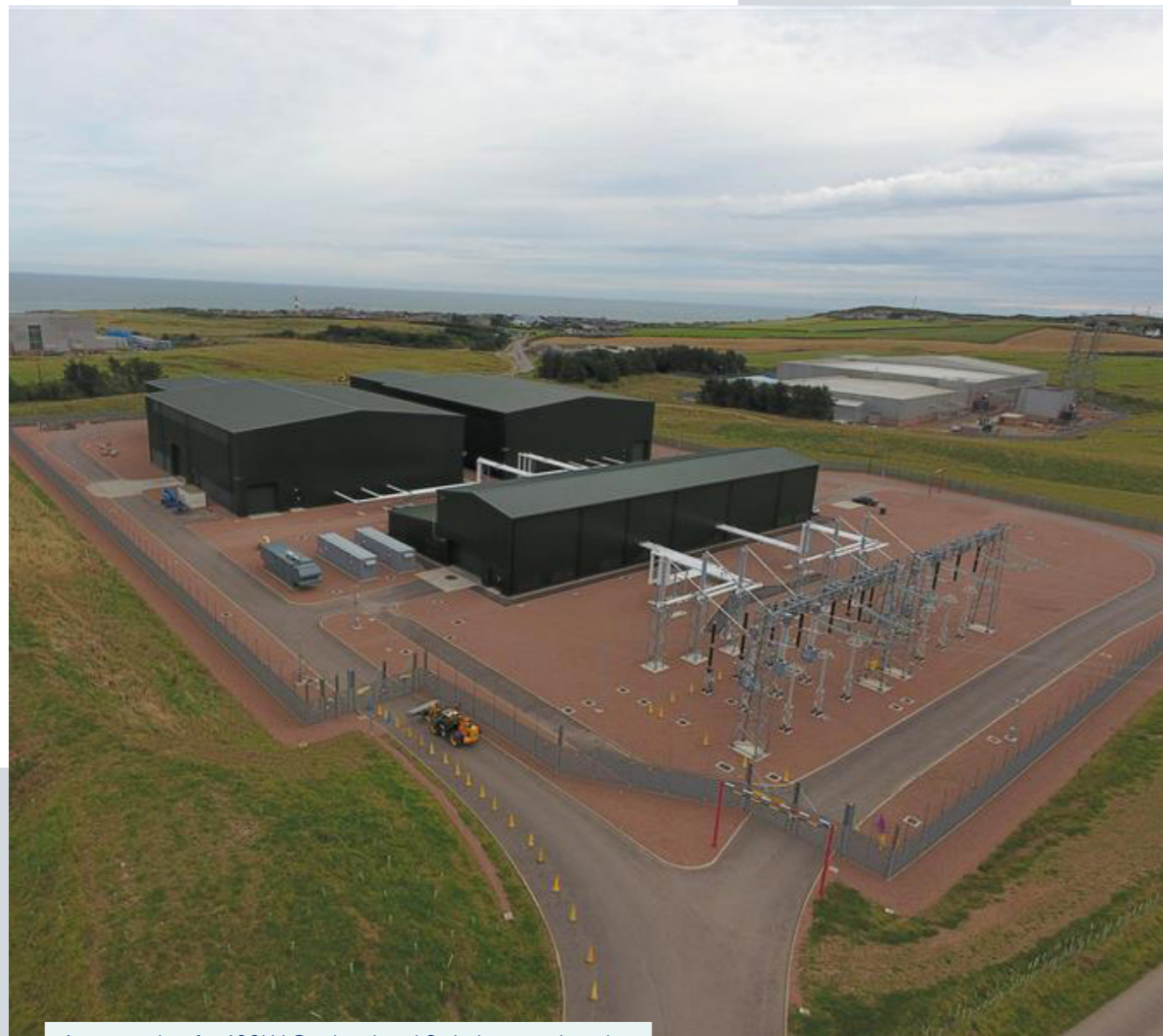
An example of a 400kV Gas Insulated Switchgear substation
