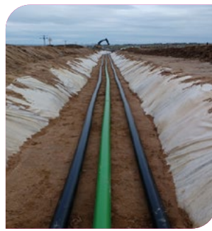
UGC power cables; either ducted or directly buried, in an underground trench nominally 1m below ground level.
