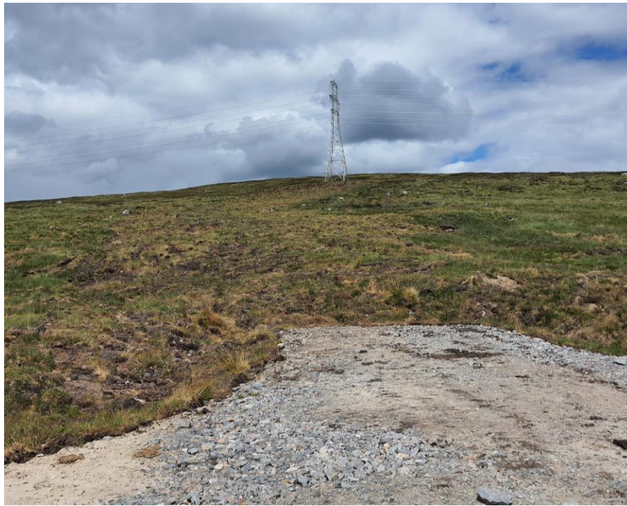
Photo 5: Reinstatement of temporary access track to tower and narrowing and reinstatement around permanent access track.
