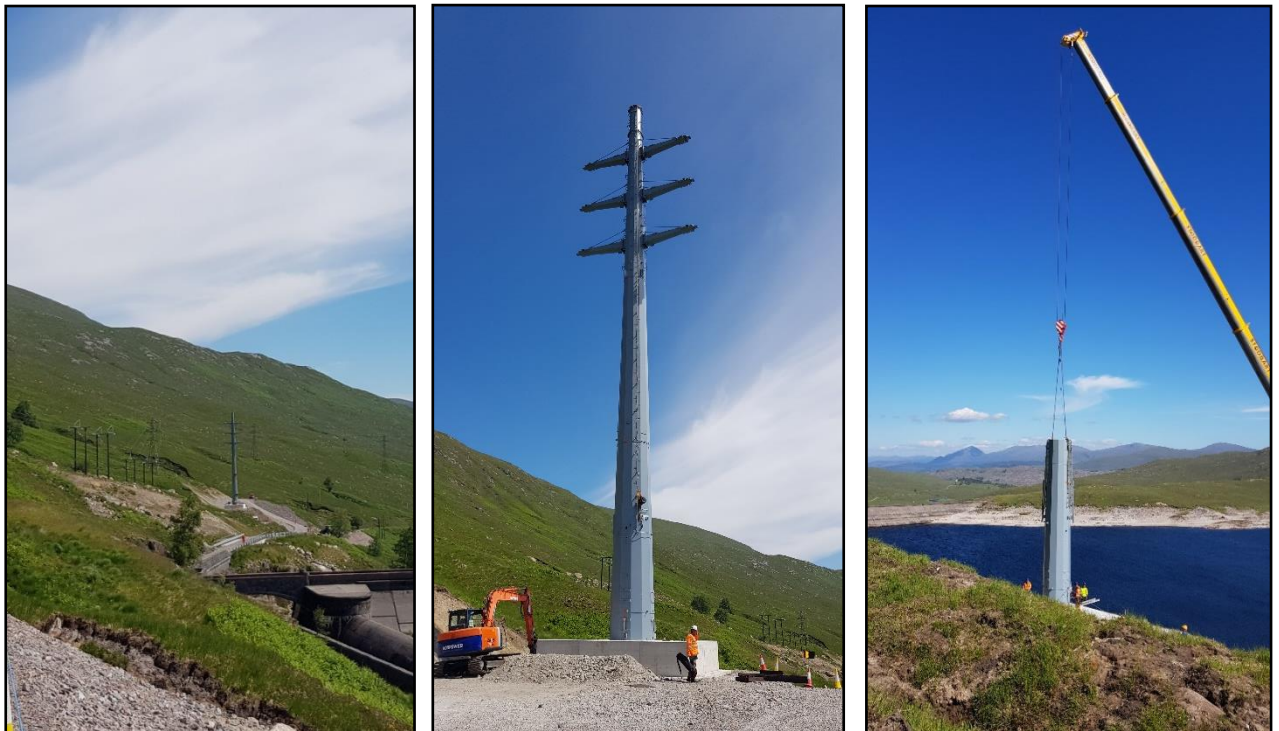
Plate 1.1: Example of NeSTS pole with larger 400m+ spans
