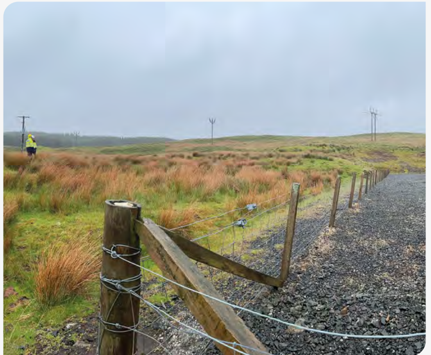
Eastern fenceline of the existing substation
