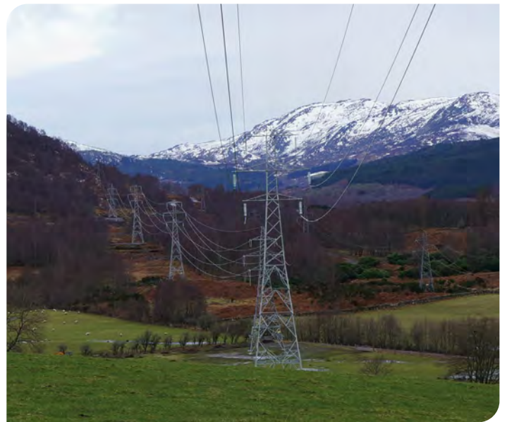
Figure 2 An example of a Steel Lattice L7 Tower Structure
