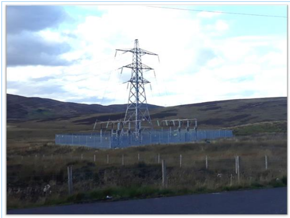
Plate 2.7: Example of a Cable Sealing End Compound
