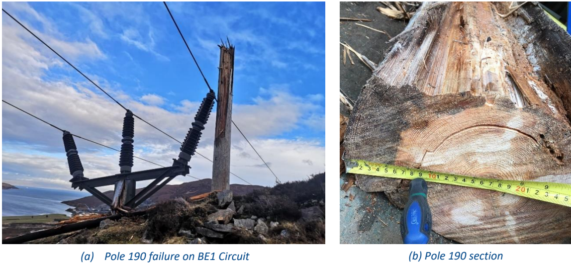
Figure 8. graphic details of the failed pole 190 on BE1 line on 23 February 2021
