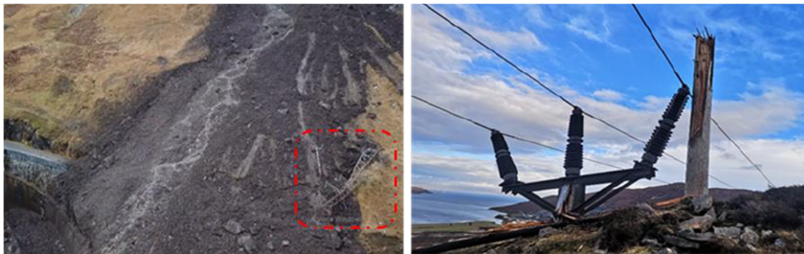
Figure 5. a) Landslide in 2018 with toppled steel lattice tower highlighted, and b) 2021 wood pole failure
