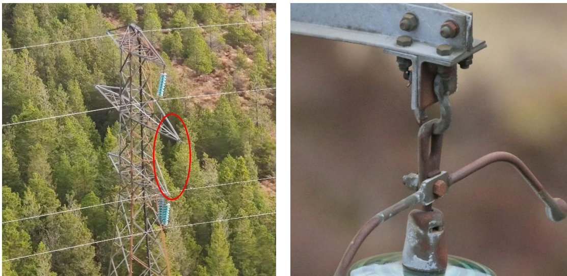
Figure 7. a) Tower 92 QB1 Circuit Middle Phase Shackle Failure and b) example of similar Shackle and point of Failure showing Extreme Wear
