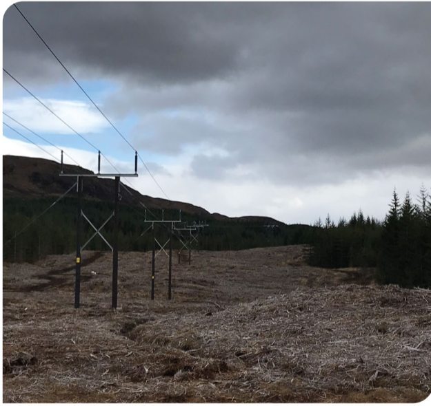
Figure 1 An Example of a Trident H wood pole structure
