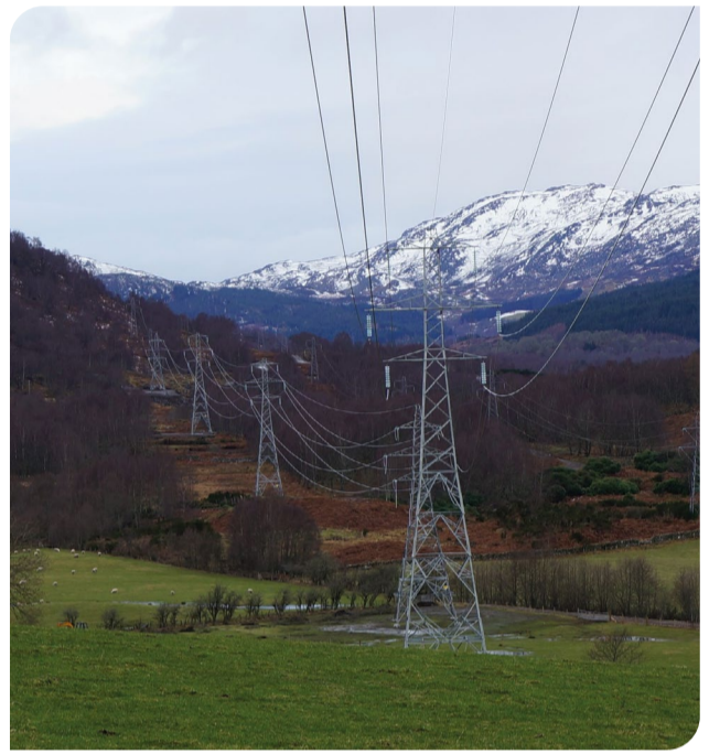
Figure 2 An example of a Steel Lattice L7 Tower Structure
