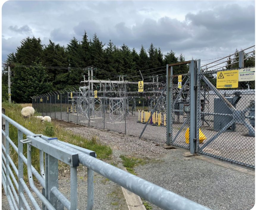
Existing Broadford Substation looking eastwards
