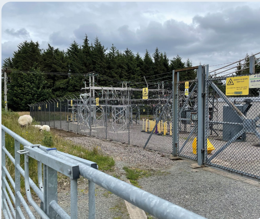
Existing Broadford Substation looking eastwards
