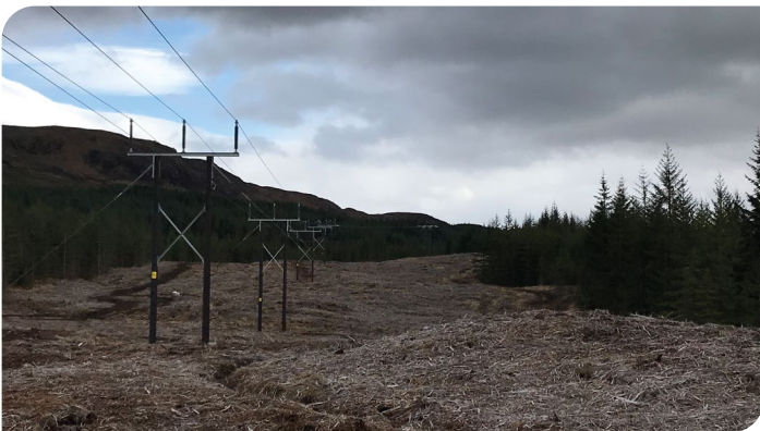
Figure 1 An Example of a Trident H wood pole structure
