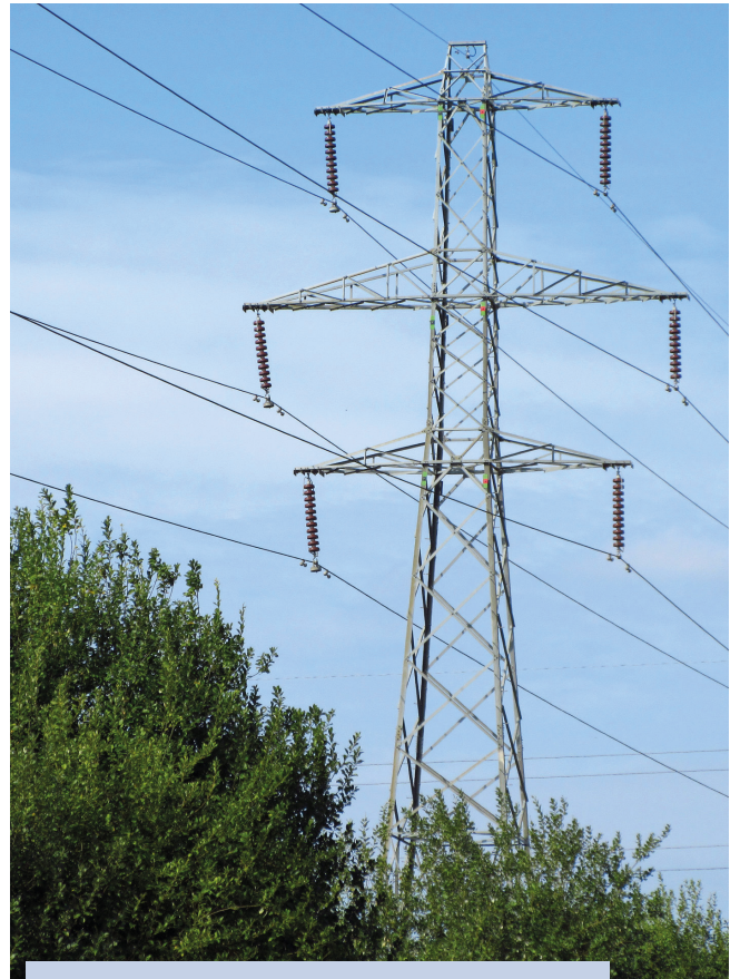
Steel lattice tower double circuit (L7 series)
