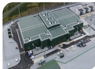
Operational 1200MW Blackhillock HVDC Converter Station.
