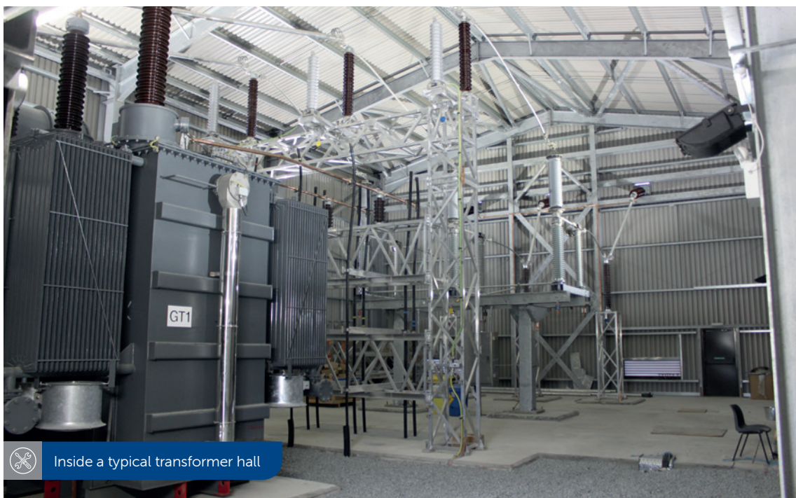
Typical 132kV Transformer hall
