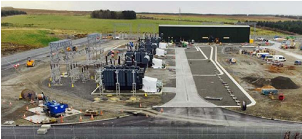
Caithness Moray - Spittal AC substation with SGTs in the foreground and GIS building to the rear
