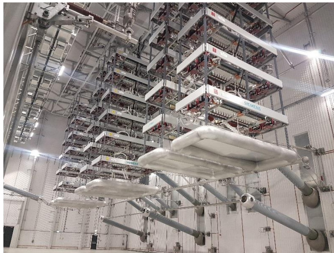
3 – Thyristor valve hall, part of HVDC systems used in subsea links. Outages on transmission equipment are required for maintenance to keep the network safe and reliable as well as to carry out upgrades to increase capacity
